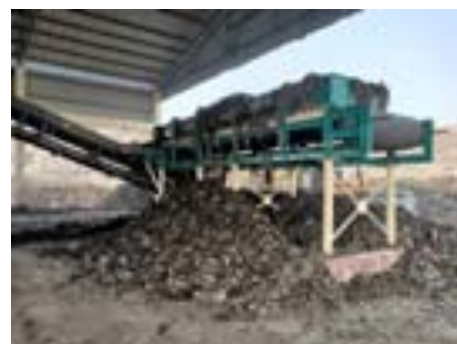
Figure 4-76: Treatment facility in Bakarganj SWM plant
