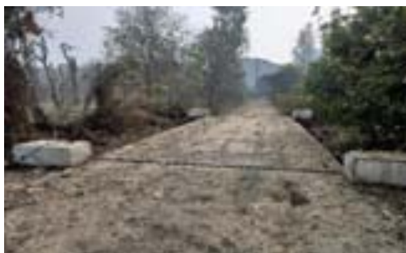
Figure 4-74: Abandoned approach in Rajau Paraspur SWM Plant
