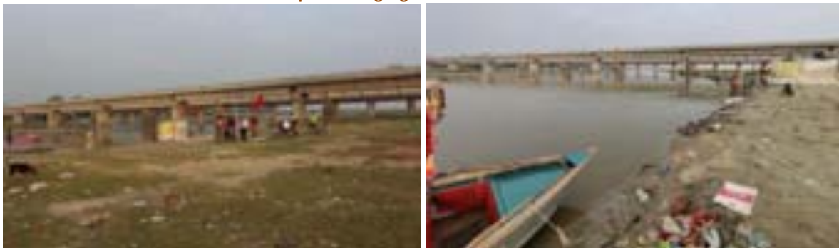
Figure 7-5: Dilapidated Ghat along river edge and connecting bridge (left), Vacant Land Parcel near bridge (right)
