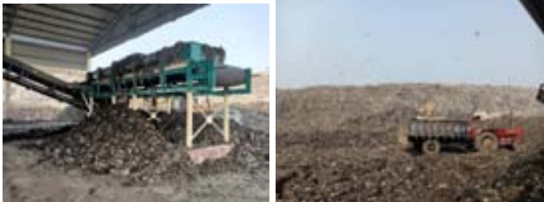
Figure 5-103: Dumping yard in Bakarganj SWM plant (left) Treatment facility in Bakarganj SWM plant (right)
