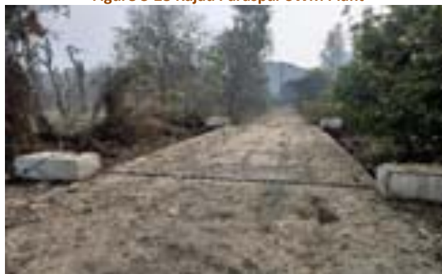
Figure 3-29 Abandoned approach in Rajau Paraspur SWM Plant
